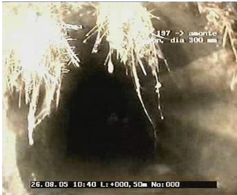
Fig. 1. Root intrusions in concrete sewer pipe [1], [2]. The roots are starting to branch already.
