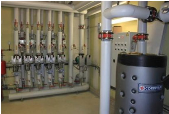
Fig. 3. Technical room (MORBIHAN ENERGIES).
