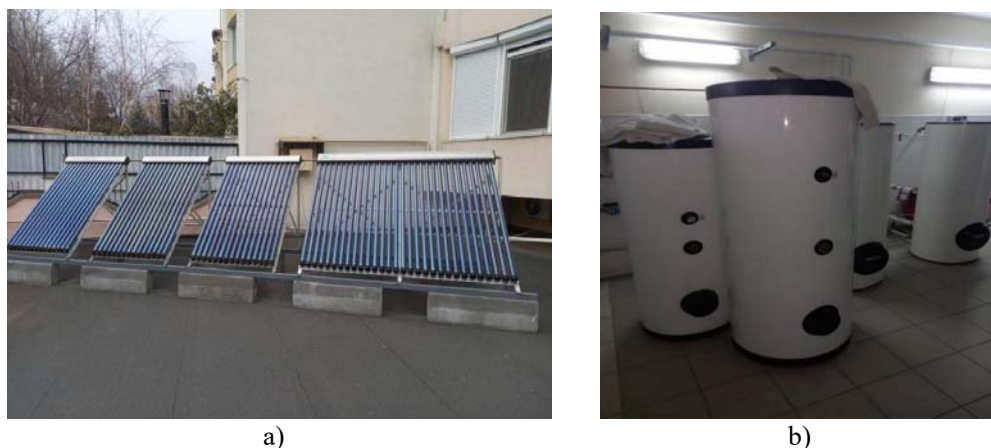
Fig. 3. a) Solar panels with vacuum tubes for the preparation of DHW b) Boilers with 2 coils for DHW preparation
