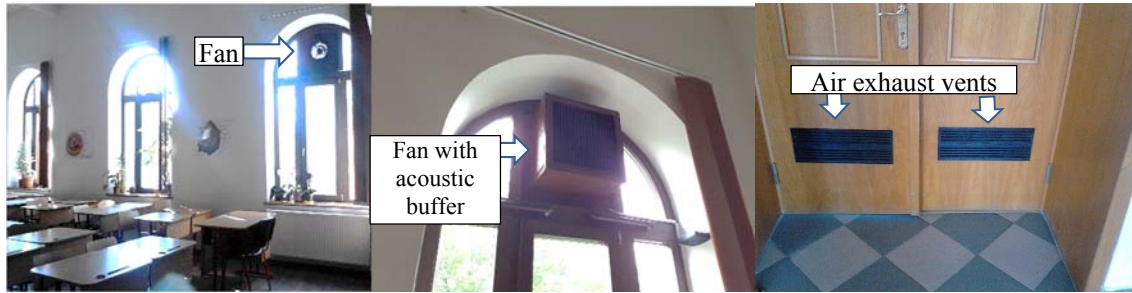
Fig. 3. Photos of the ventilation system
